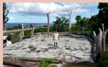
Farea cyclone shelter, Mangarisu village, Tongoa, Vanuatu in 2010 (upper) and after Cyclone Pam in 2015
