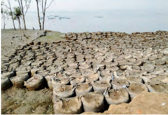
Figure 6 Sandbags for mitigating river erosion (Photo: S.K. Abdullah Al Mamun)
